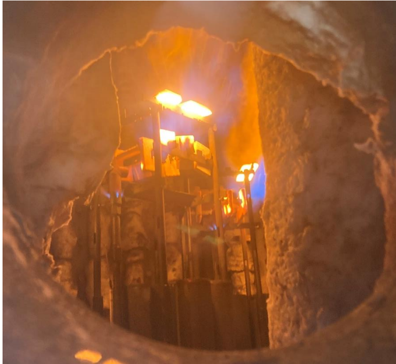
Figure 4 - Photograph of multiple burners operating in the Increased Throughput, Compact Flame Application
